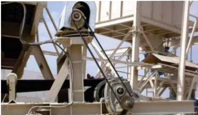
Conveyor in a Stone Crusher Plant
