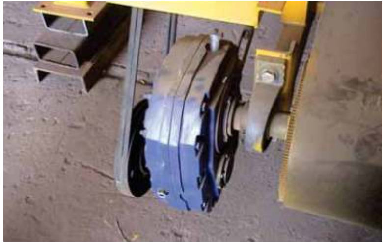
Conveyor Belt Drive
